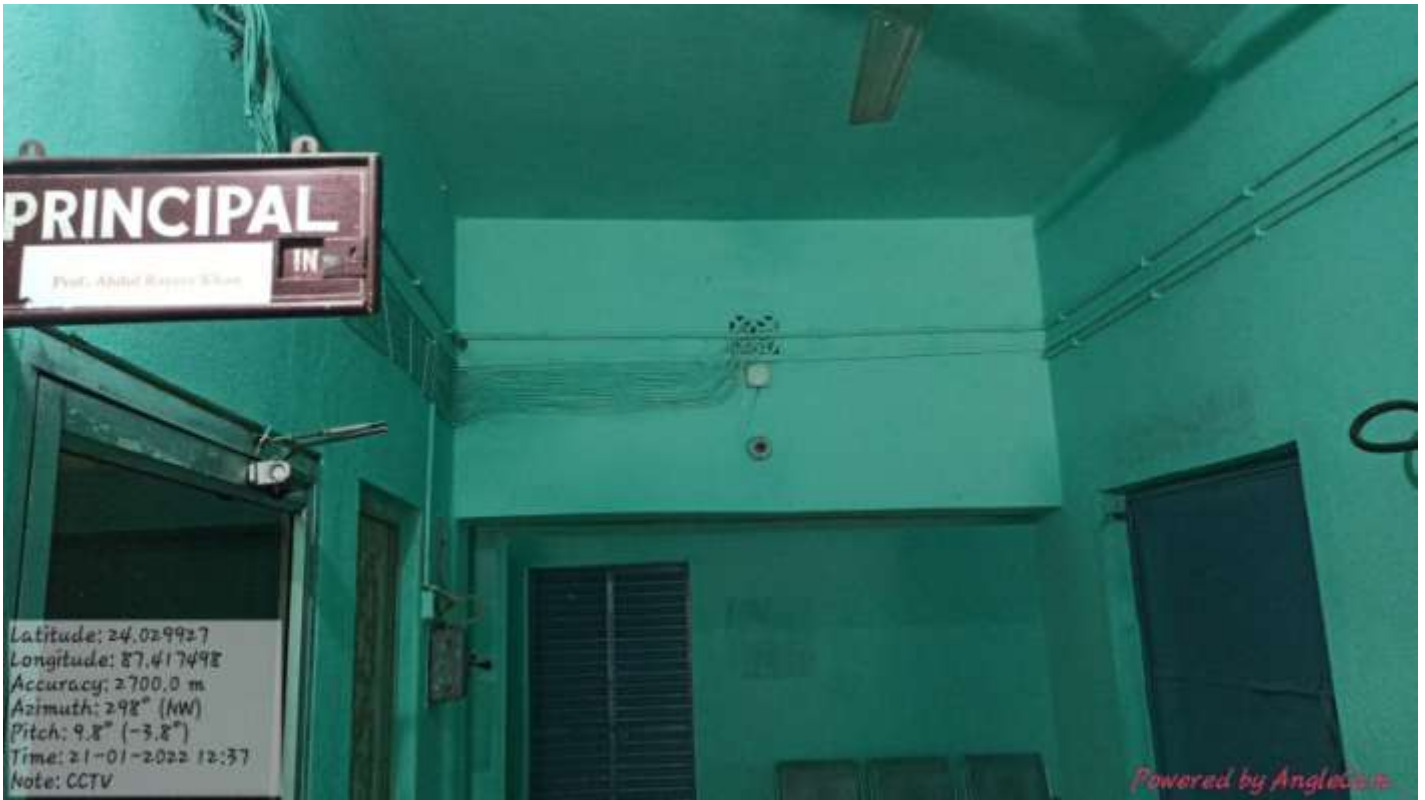
Fig. 1 CCTV camera in corridor
